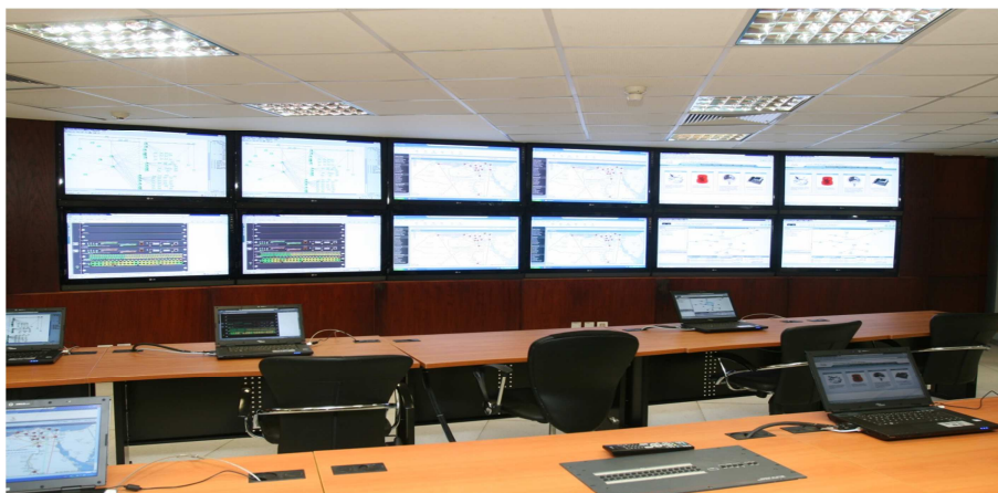
Figure 11: Network Operation and Monitoring Center
